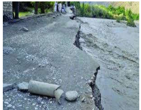
Figure 15: Flooded stream, Dir
